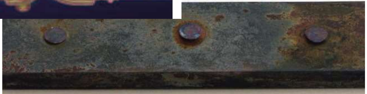
Copper rivets on a steel bar submerged in 3% sodium chloride solution after ten months
